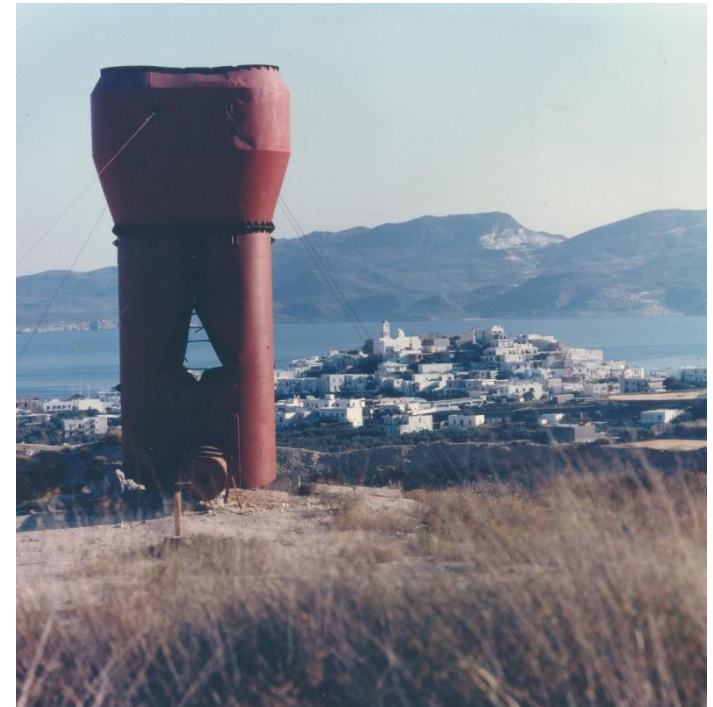
The steam separator of Milos geothermal power plant and village of Plaka
